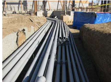
Building A Electrical Room Conduits
